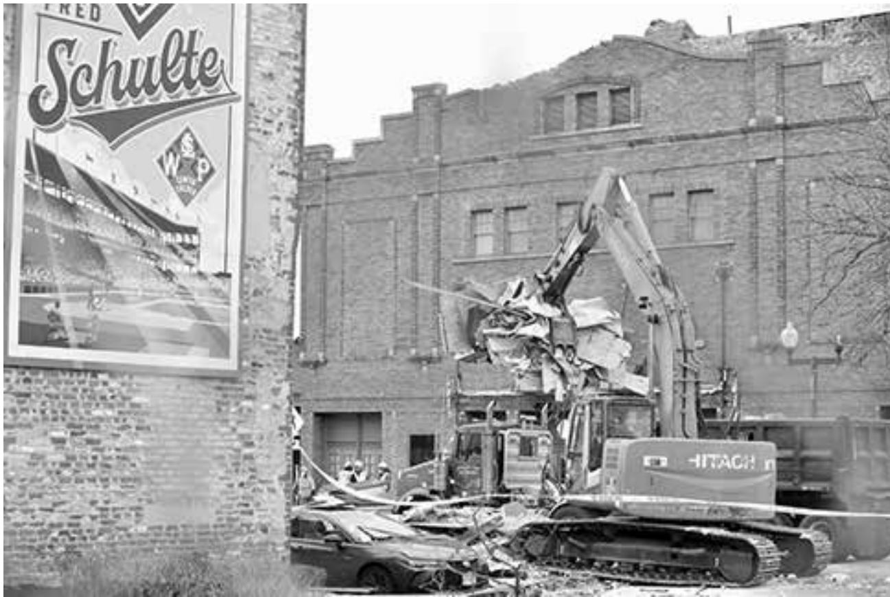
Clean-up of debris from the tornado
