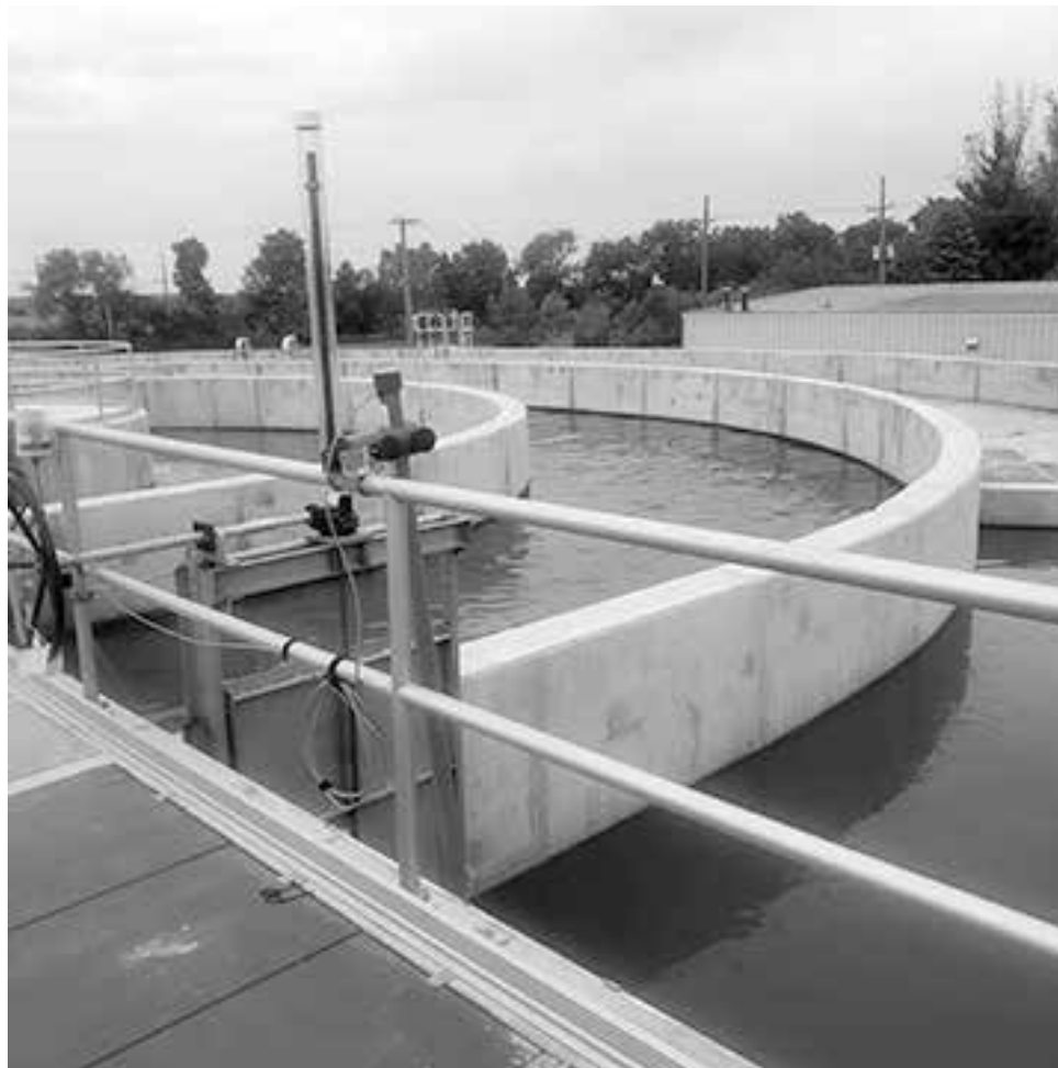
New digester has three rings
